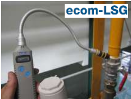
Pressure test on gas valve train
