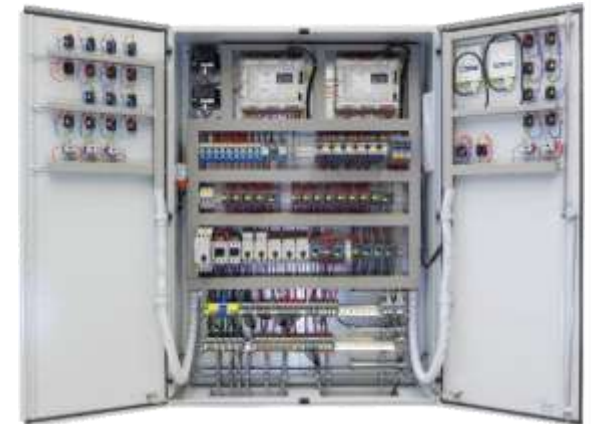
Weishaupt control panel with two W-FM 200 combustion managers
